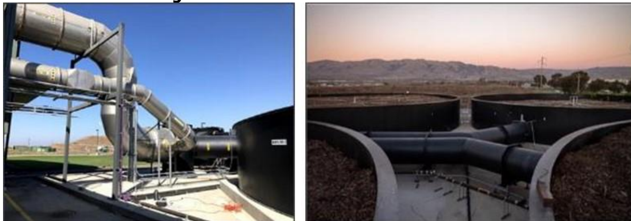
Figure 27: Acid Scrubbers and Biofilters
