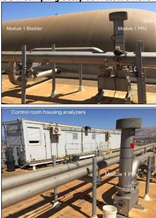
Figure 34: Sampling Setup at Pressure Relief Valve
